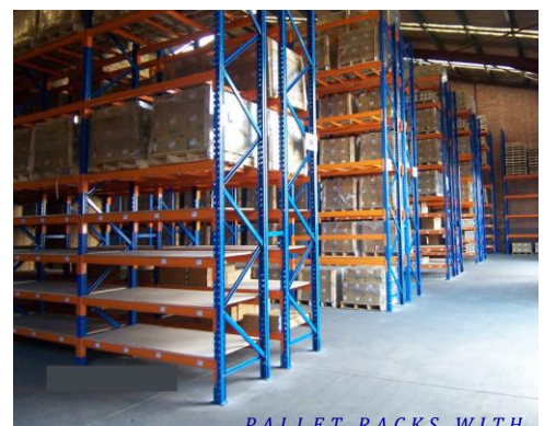
PALLET RACKS WITH PICKING SHELVES
